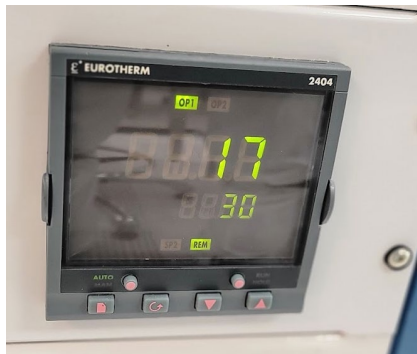
Figure 8. Temperature controller set to 30C
