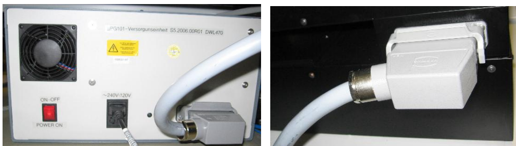
Figure 7: System power connection from supply unit (left) to lithography system (right)
